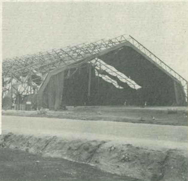
caused considerable damage to our big hangars.
