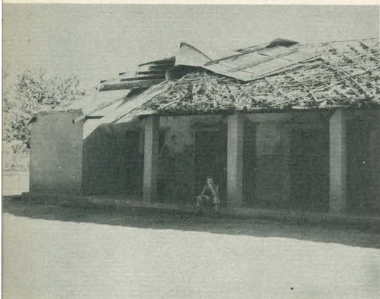
Storms still caused some damage . . .
