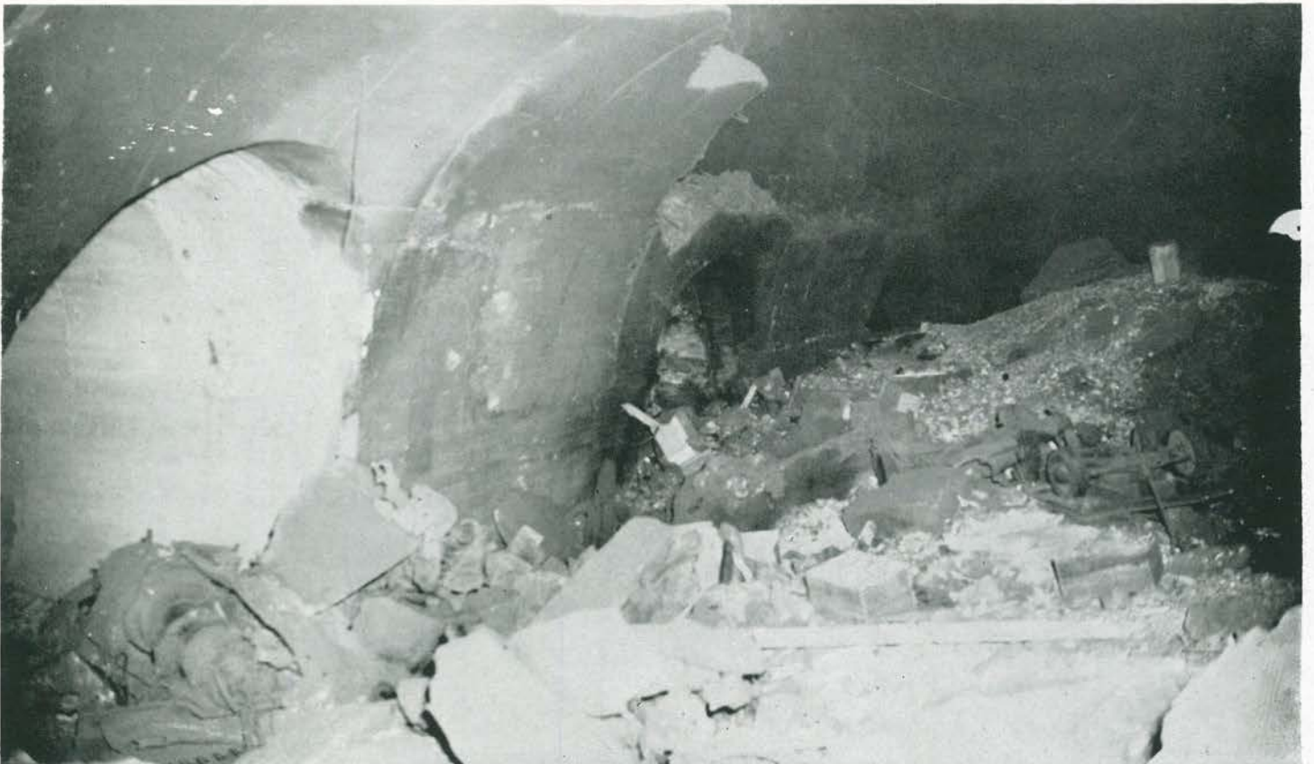
Rubble In Wainwright Tunnel
