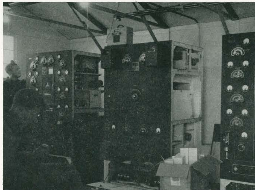
Inside Radio Building, Installing Transmitters
