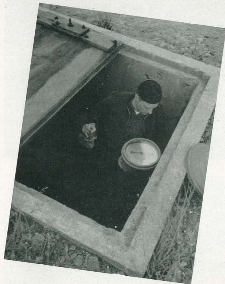
Portion of Aqua System and Operator
