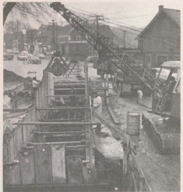
Davis Brook Trunk Sewer
